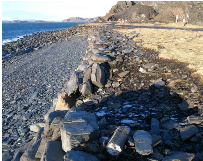
One of the areas of damage
